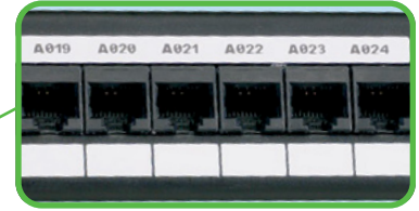
Patch Panel / Face Plate Labels
