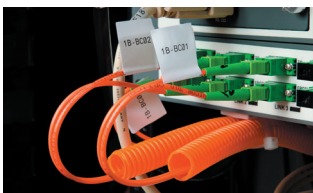
Fiber optic cable markers
