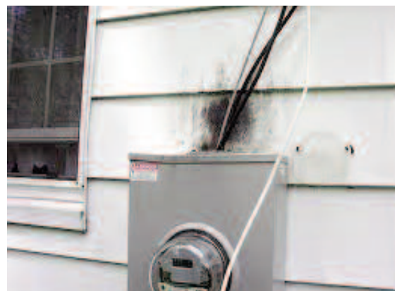
Service Entrance Destroyed By Overvoltage
