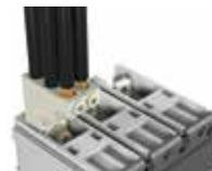
Multi-cable terminals with cables
