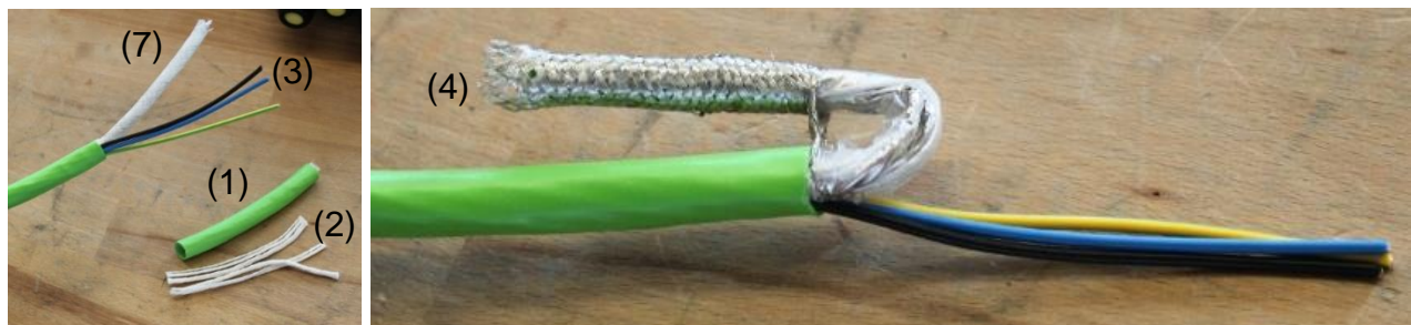
Figure 2.2 – Stripped cable and bare shielding
